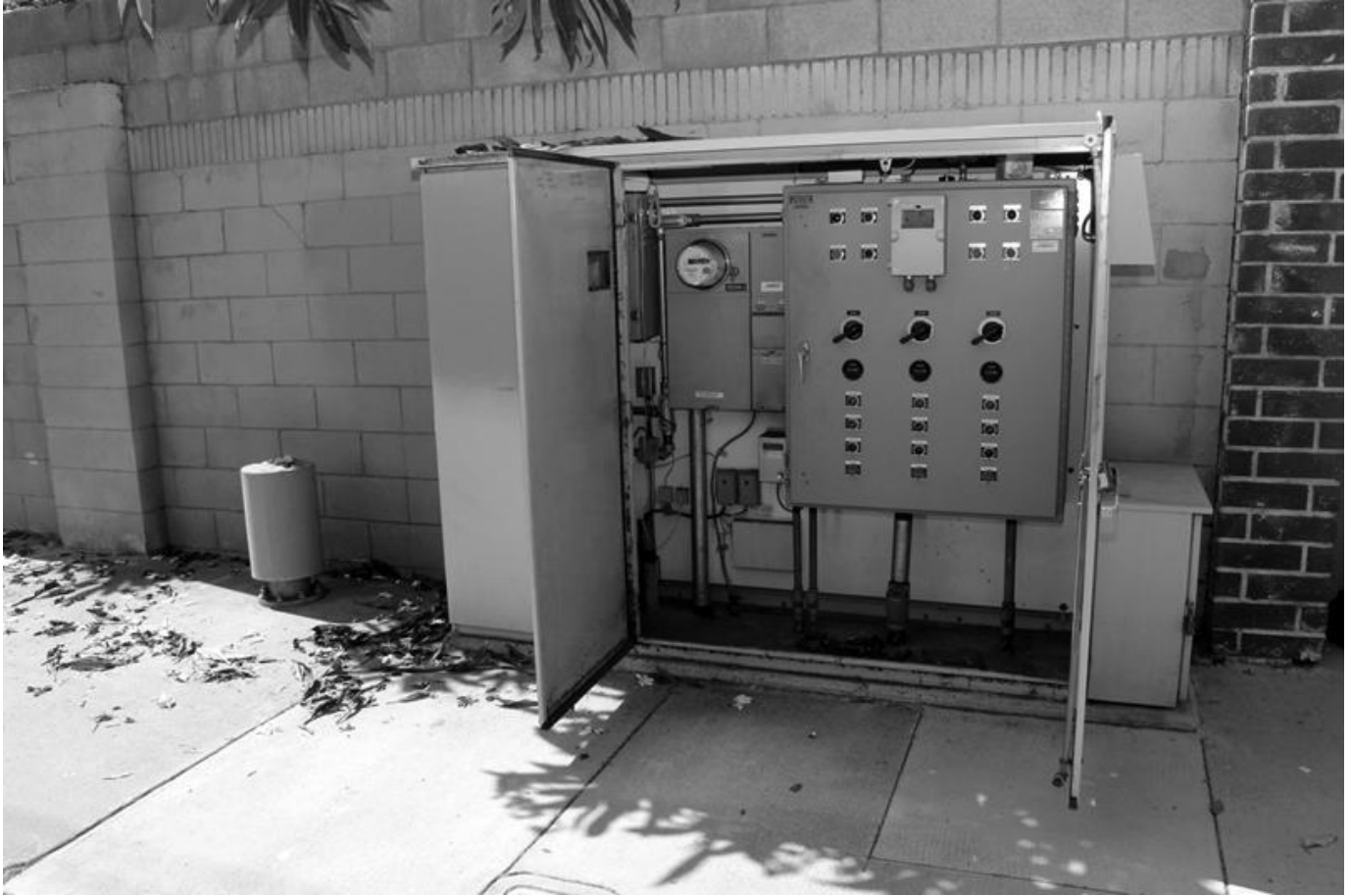
Cerritos Sewer Lift Station Control Panel
